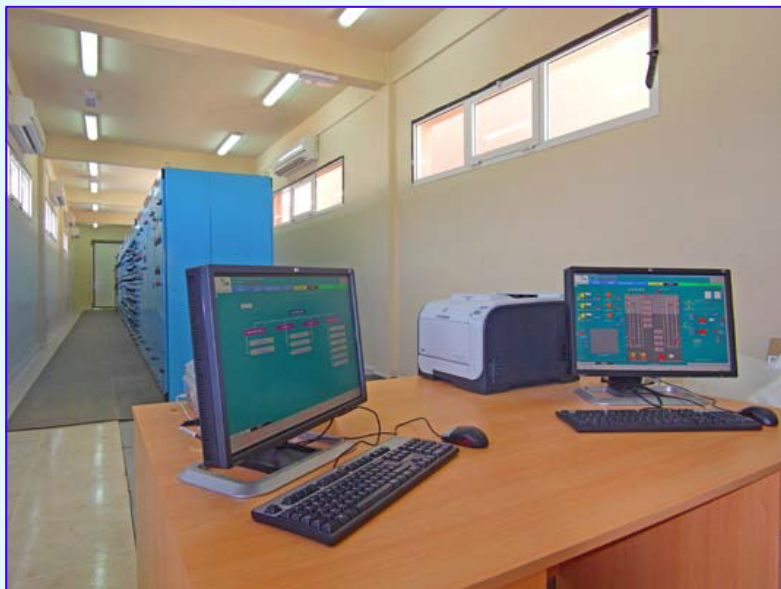
Typical Control Room on Larger EfloMBR Plants
