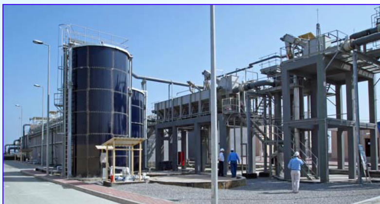
Typical View of EfloMBR Inlet Works, 6 + 3 mm Screens, FOG & Grit
